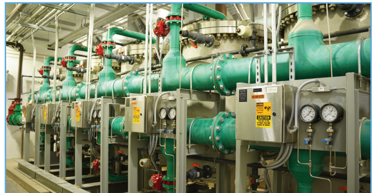
Stonytown Well 10 Station is near completion and blends in perfectly within the local community. The ion exchange for nitrate treatment has been installed and is fully operational.
